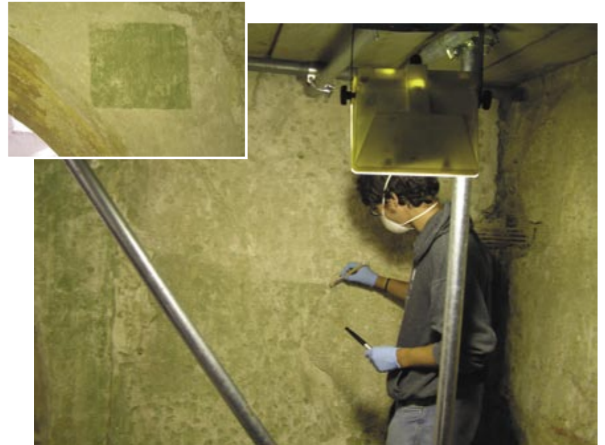
Figs 24: Careful removal of green micro-biological growth during conservation (Inset) Fig 25: Test area showing the difference between cleaned areas and green square of micro-biological growth
