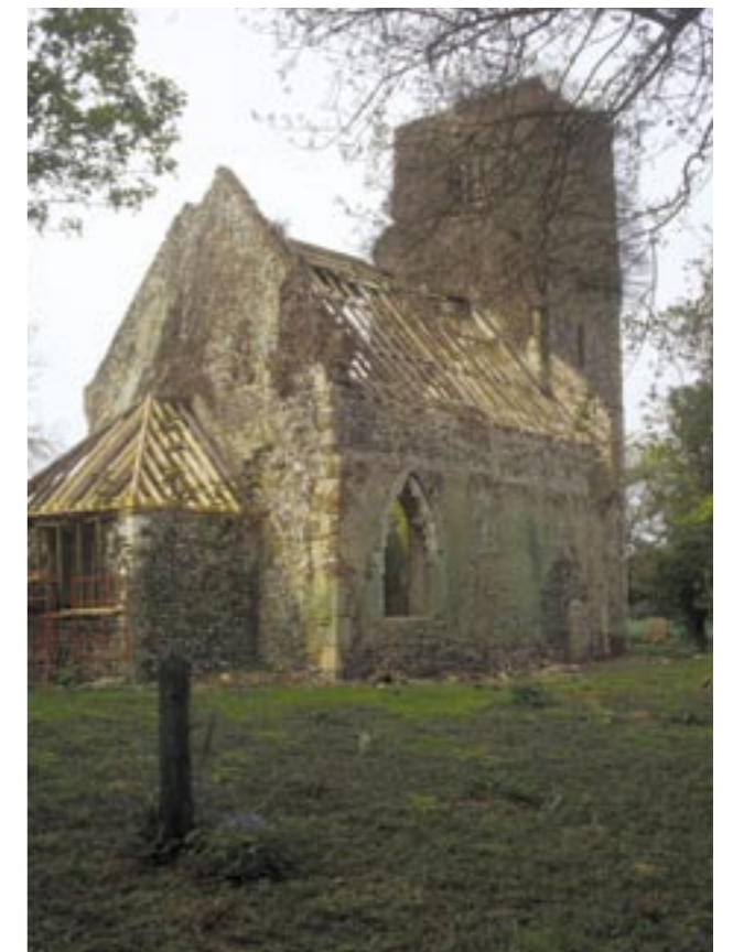
Fig 17: Repairs to the roofs under Norfolk County Council's Ruined Churches Repair programme in the 1990s
